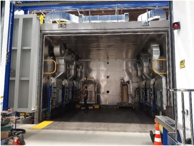
Fig. 1. Production plant oven A for the drying process
